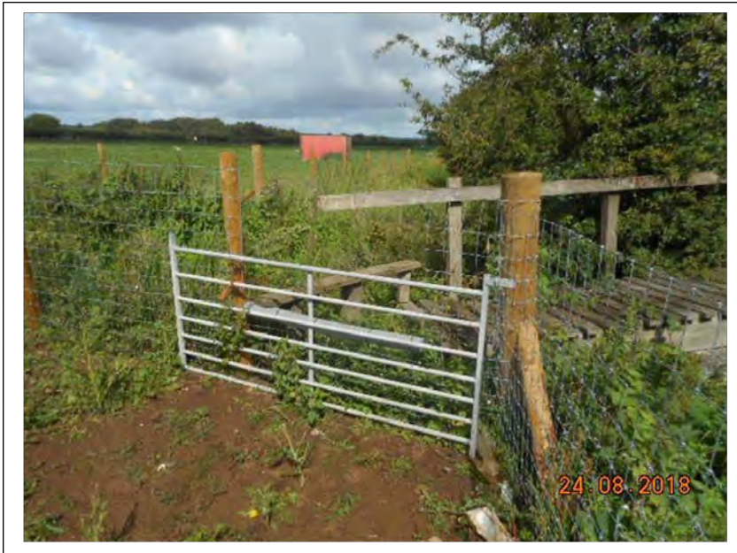
Image 20 shows missing stile, stile out of repair, landowner responsibility.
