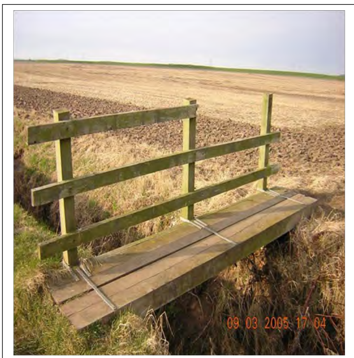
Image 16 damaged handrail report to Structures, Development and Design .
