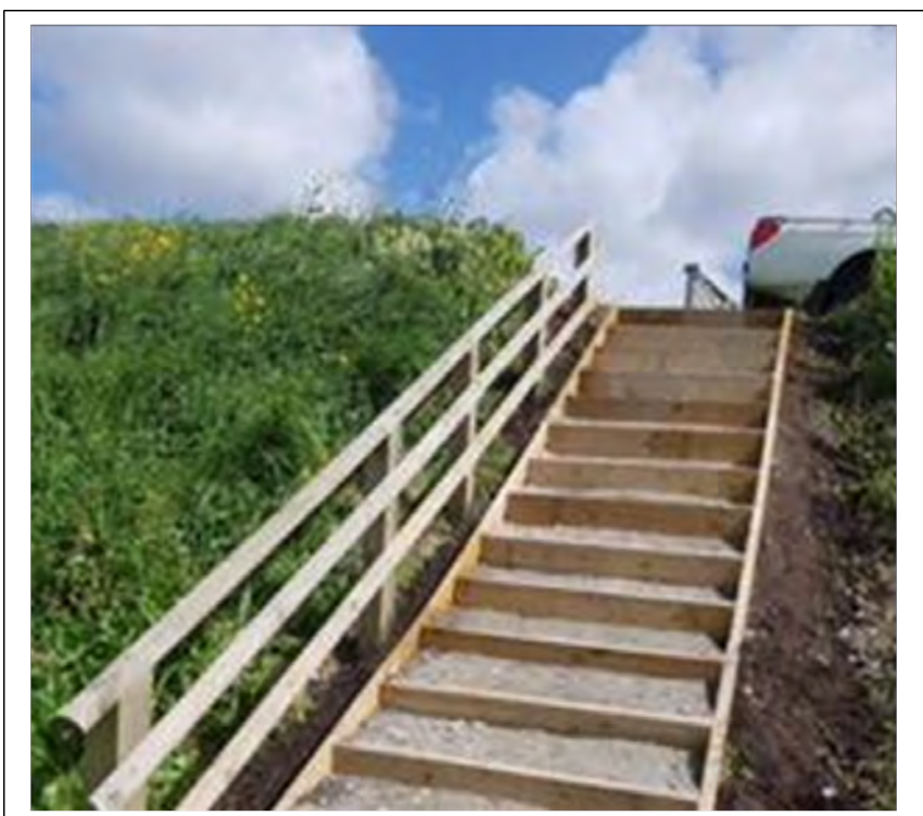
Image 19 show repaired damaged steps Ince Blundell Footpath Number 6; this defect presented a danger to the public.
