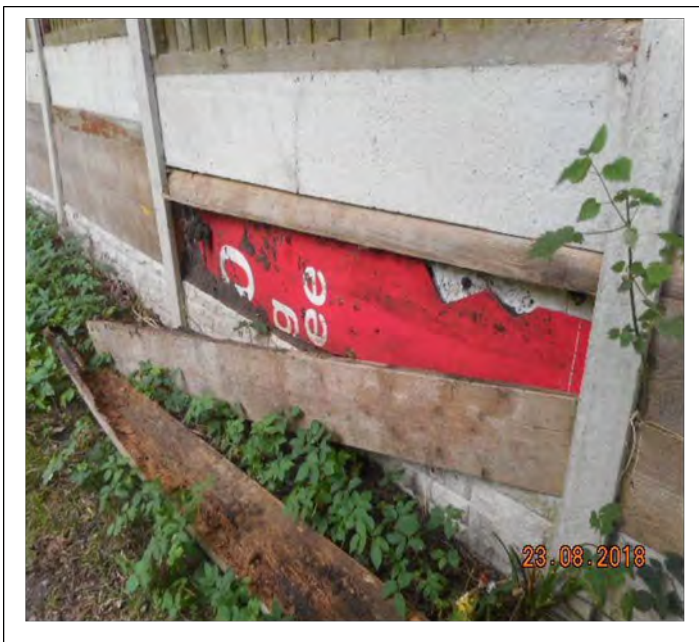
Image 2 dangerous structure adjacent to PRoW report to Highways Enforcement .
