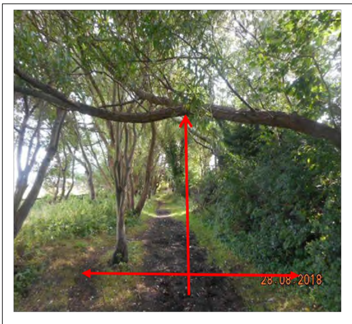
Image 26 Bridleway low tree branches need to be cut at a minimum height of 3.5m from ground level minimum width of 3m Grounds Maintenance HM5 contract.
