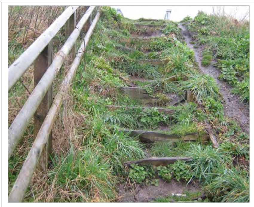
Image 18 show damaged steps Ince Blundell Footpath Number 6, this defect presented a danger to the public.
