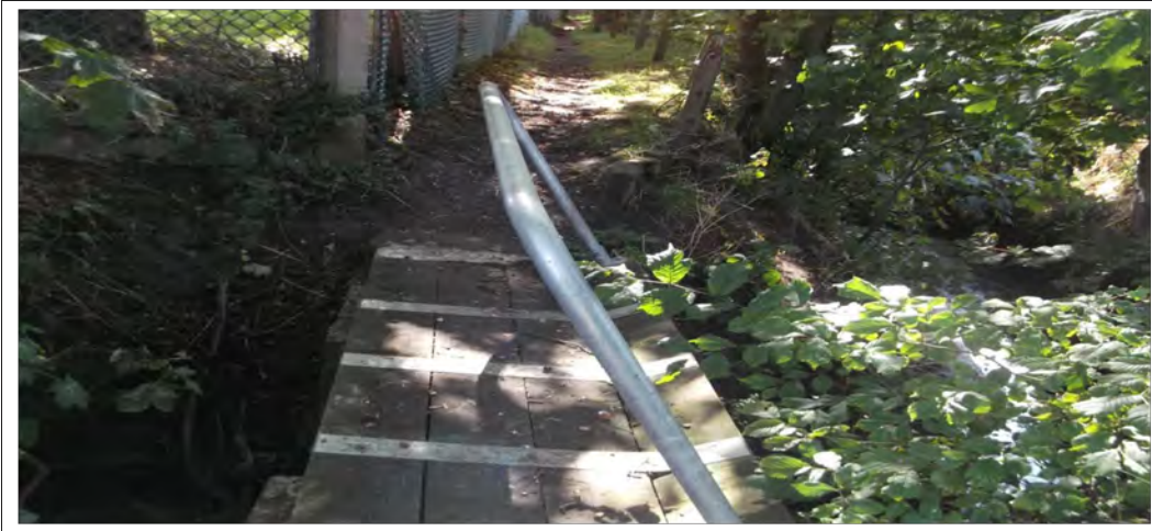
Image 15 Damaged handrail Melling footpath No. 11, report to Structures, Development and Design.
