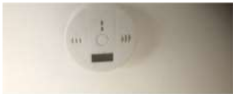
Smoke detector fitted
