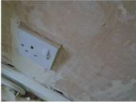
Socket identified in bathroom
