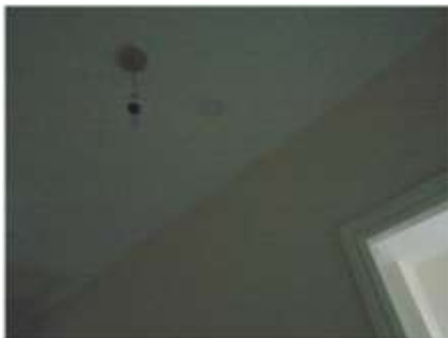
Missing smoke detector
