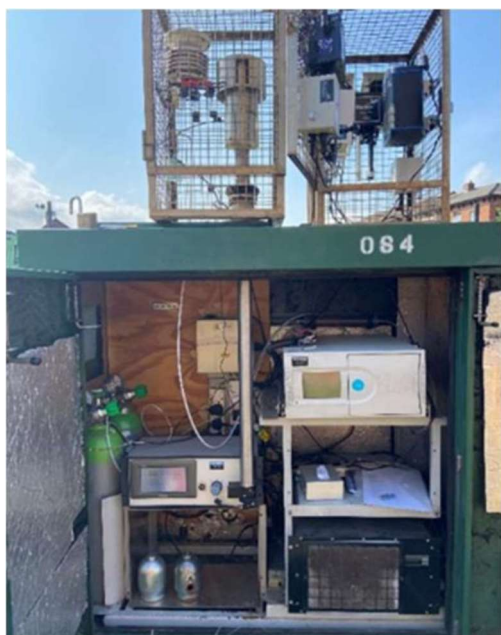
Picture - Co-Location of Sensors at Millers Bridge Monitoring site
