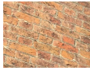
St. Peter's Church, same brick with evidence of weathering
