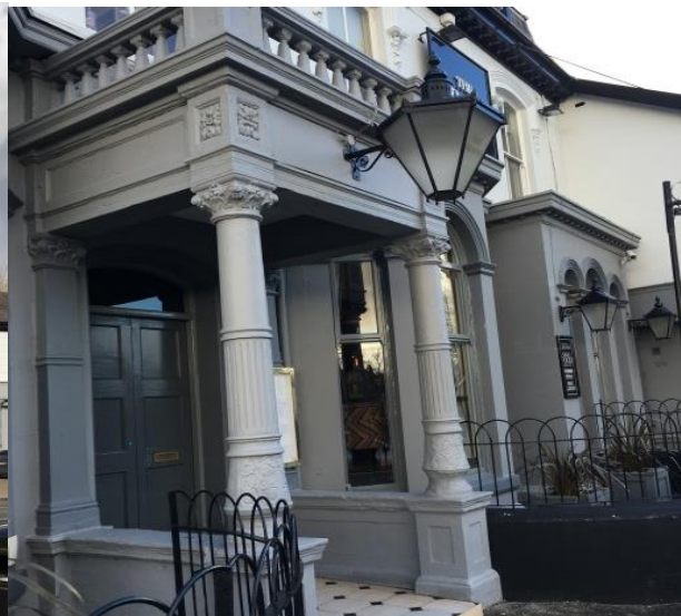
Decorative elements of The Grapes Hotel have recently been restored. The rendering has been altered significantly although it remains aesthetically pleasing
