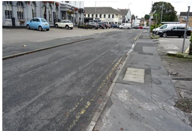
The pavement on Green Lane adjacent to the Embassy Building and Grapes Hotel shows significant signs of wear and lack of maintenance (Photo October 2019)
