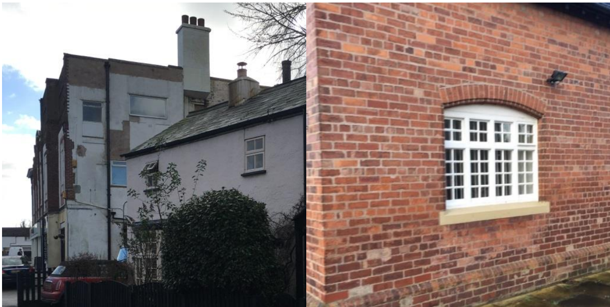
The north facing elevation of the Embassy Building looks into the Conservation Area and its poor condition is extremely detrimental to the character of the building and area as a whole
