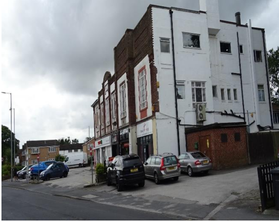
The appearance and general condition of the north façade of the Embassy Building is at odds with the character of the area (photo July 2019)
