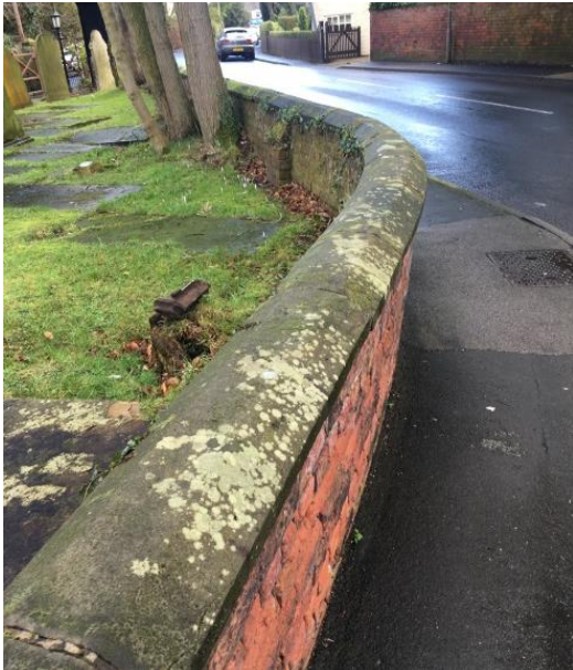
The boundary wall to St. Peter's Church shows signs of weathering. However, is generally in good condition
