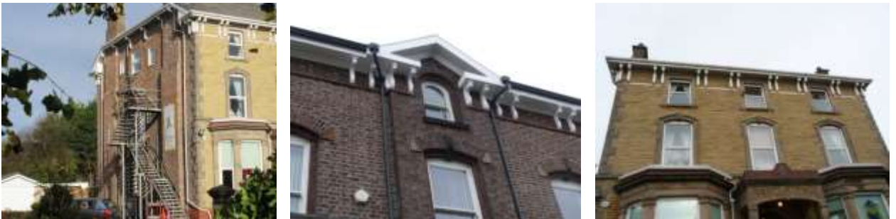
A variety of double eaves brackets found throughout the Christ Church Conservation Area
