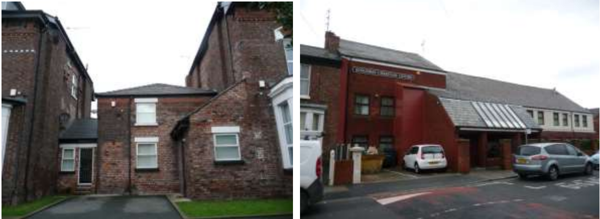
Examples of detrimental 'linking' and inappropriate extensions found within the Conservation Area
