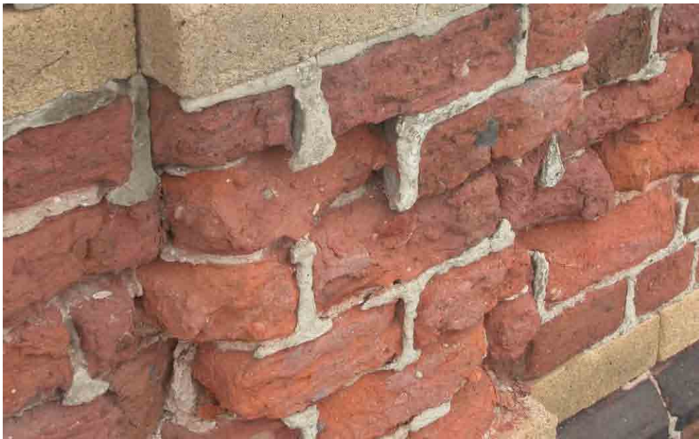
The dramatic effects of hard pointing on soft brick
