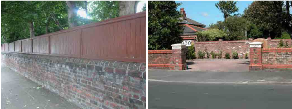
(left) fence added on top of old boundary wall; (right) driveway widened – the left hand gate post has been carefully moved.
