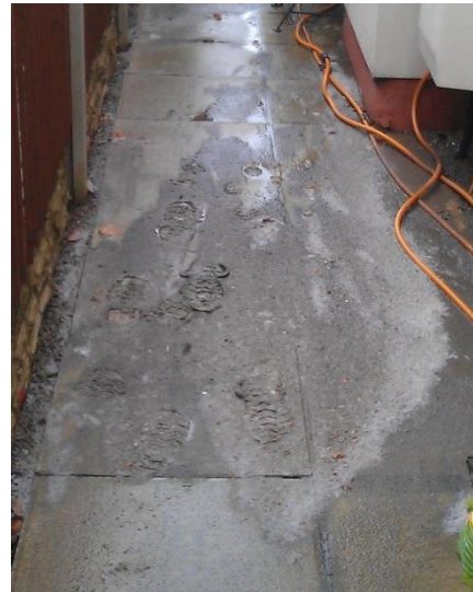
Figure 5: Foul debris residence side passage
