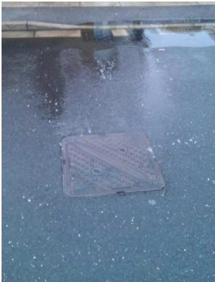
Figure 4: Toilet type debris emanating from a drain in the road
