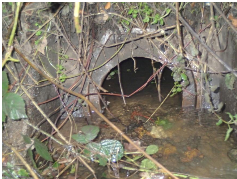
Figure 8: Outfall from Fouracres into Whinny Brook, taken 06/11/2012
